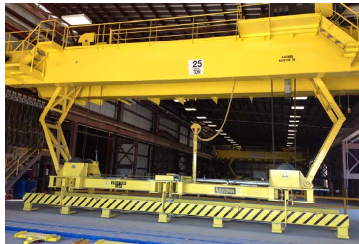
25 metric-ton hydraulic plate lifter in a steel mill is reeved directly to the crane and includes anti-sway bars.
