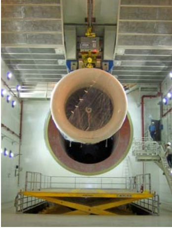
12,000 pound capacity jet engine test cell lift platform. The platform is 22 by 44 feet and vertical travel is 13 feet.
